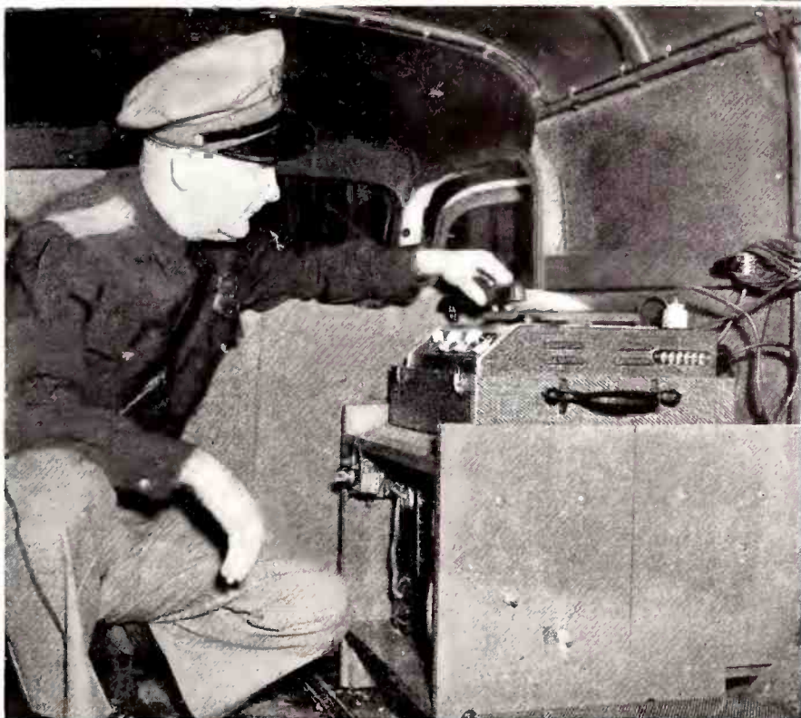
Method of mounting sound equipment in campaign truck. Note mounting rack for amplifier and cleat for cable at far right. Equipment installed by Olsen Radio Supply Co., San Antonio, Tex.
